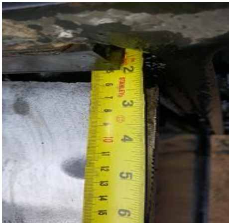
Fig 3. Fissure Length since pin separator to frame.
